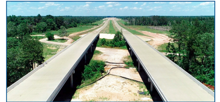
8-mile-long I-69 Diboll Relief Route south of Lufkin to be completed in the fall of 2025.
